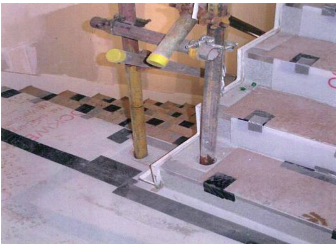
Figure 1. This photo shows cast sockets along the open side of a stairway. The sockets make it convenient to install temporary or permanent guardrails.
