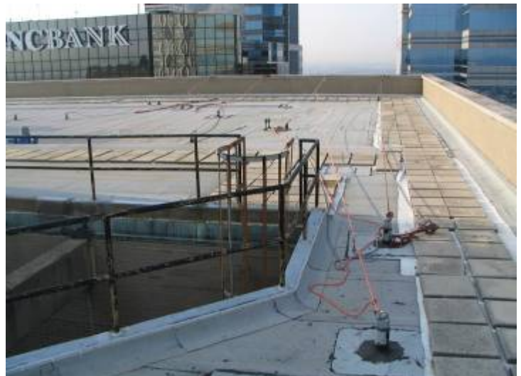
Figure 2. This photo shows guardrails installed along an opening. Installing guardrails early on in the construction process can eliminate the risk of a fall through an opening.
