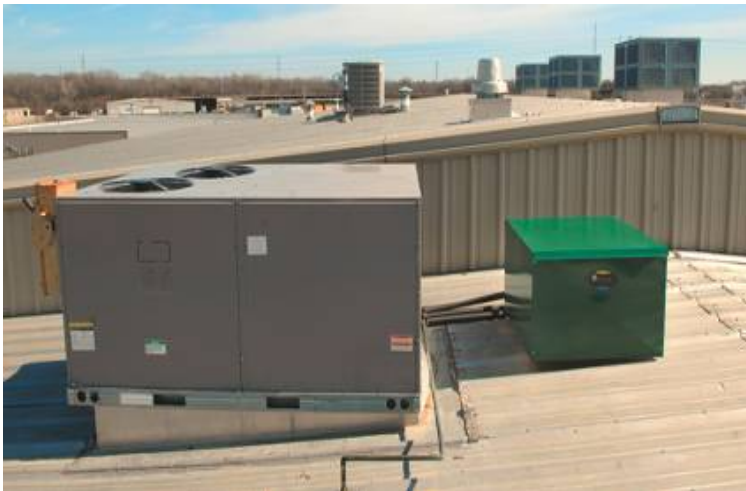
Figure 1. This photo shows equipment located on a roof. Positioning equipment at least 15 feet back from the roof edge will reduce the risk of falling when installing and servicing the equipment.
