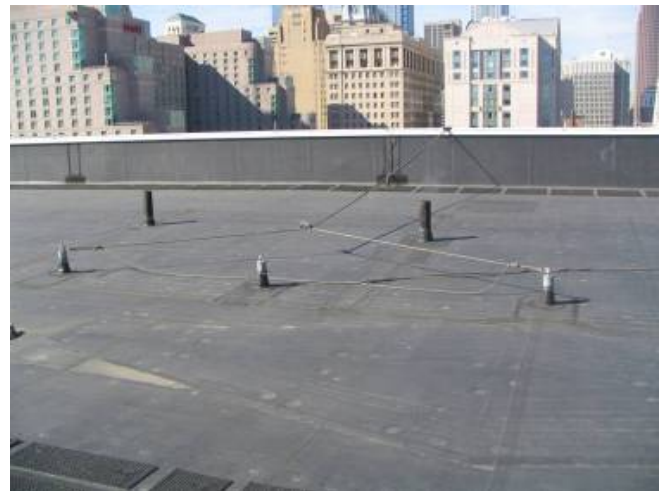
Figure 2. This photo shows permanent roof anchors. Specifying permanent roof anchors will provide convenient tie off points when working near the edge of the roof.
